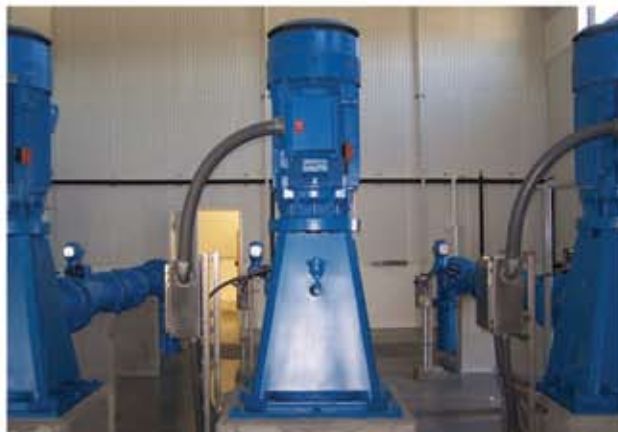
3 new energy efficient pumps/motors for the completely new Smith Street pump building
