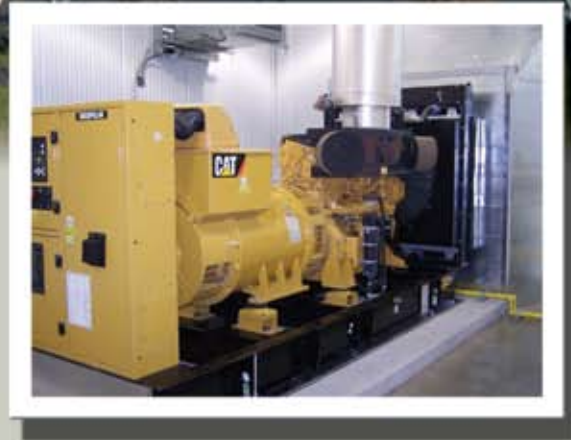
The new auxiliary power generator for the new Smith Street pumping equipment
