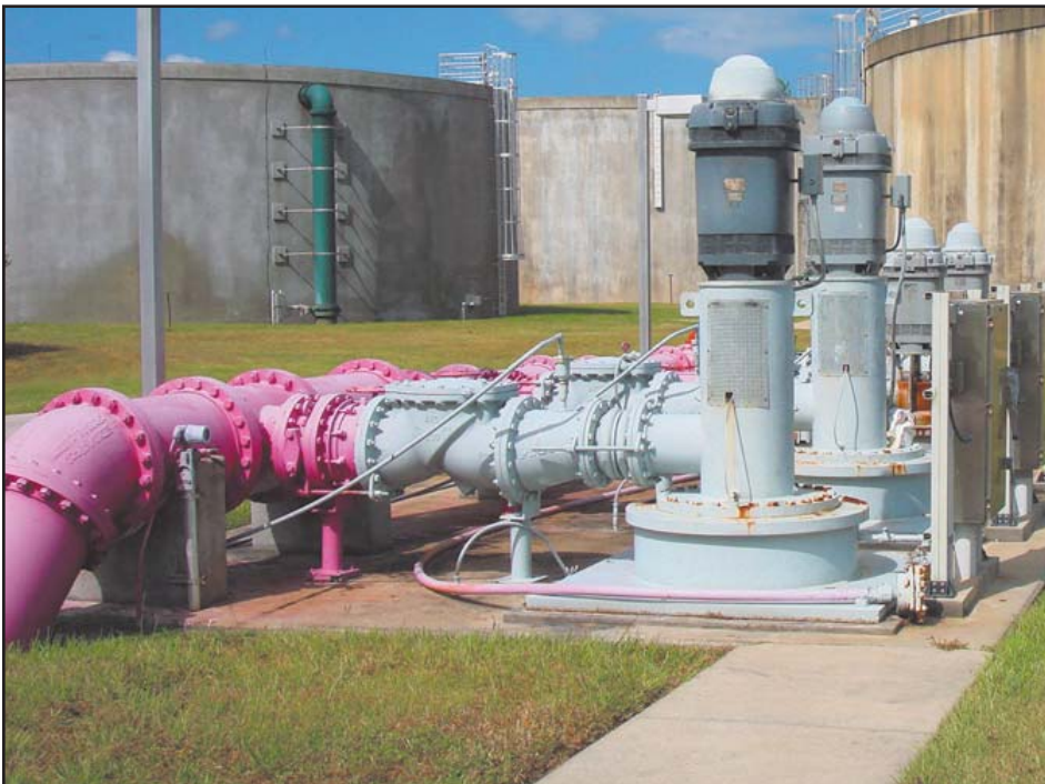
Operating these two 250-horsepower reuse distribution supply pumps at multiple settings on the VFD with slightly lowered pressure overall resulted in water conservation and energy savings that really added up.
